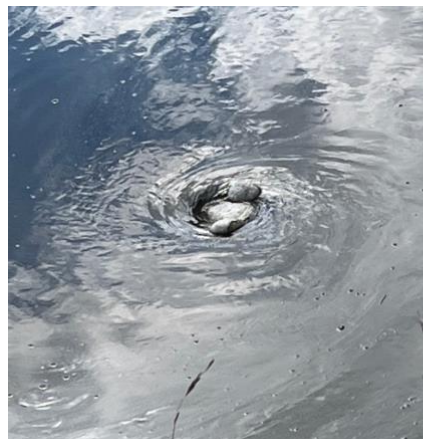
Whirlpool on the low side of an undersized culvert at Indian Rest Rd
