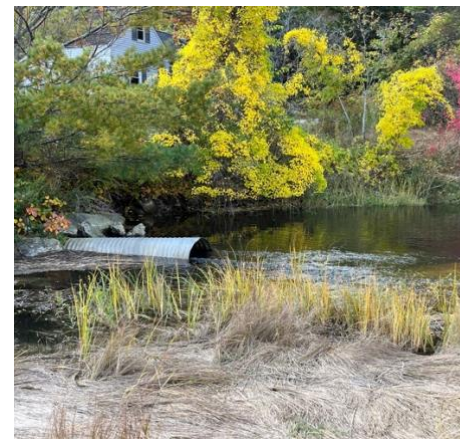
The upside of the same undersized culvert-tide coming in: culvert scour.
