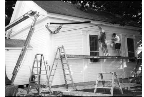
Volunteers at work last summer on the repainting of the Town Hall.
